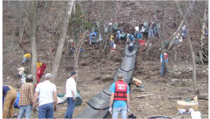
Missouri River Relief and a host of volunteers tackle the massive dumpsite on the Osage River. The flume is constructed from a culvert recovered from another clean-up event. Volunteers filled trash cans with debris and pushed them down the slide.
