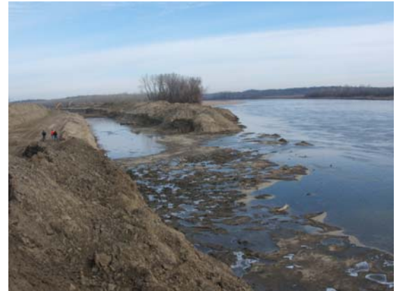
Construction of Tadpole Island chute near Columbia, Missouri to provide shallow water habitat for native Missouri River fishes.
